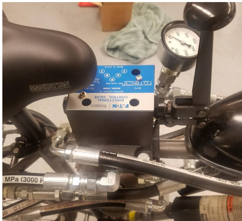
Figure 12: Directional Control Valve Placement
