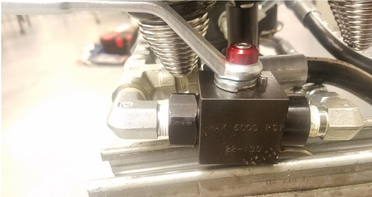
Figure 20: Ball Valve Mounted in Hydraulic Circuit
