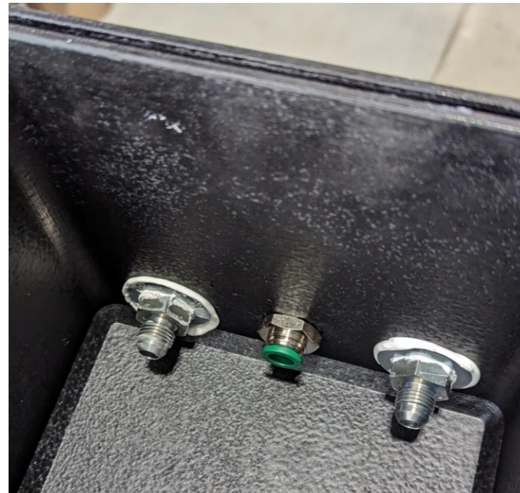
Fittings sealed with silicone
