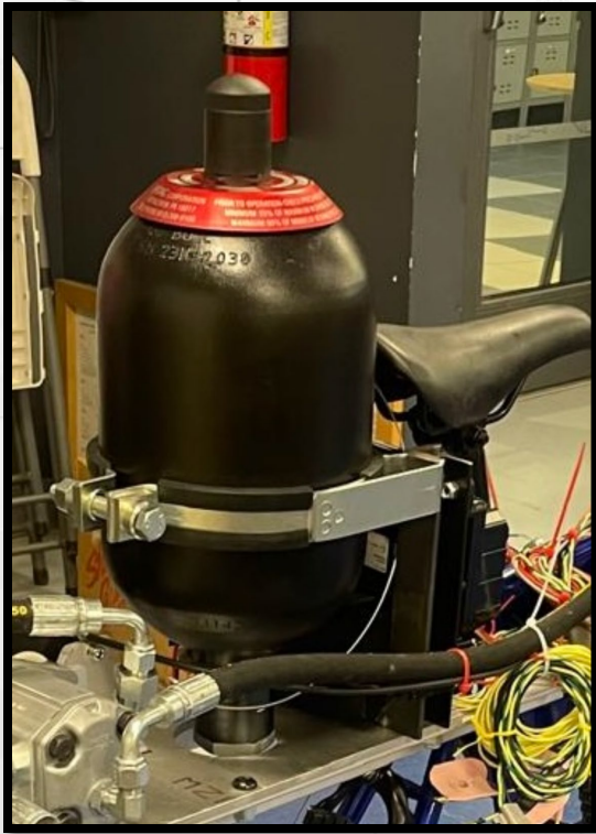
Fig. 37 Mounted accumulator PLC and battery
