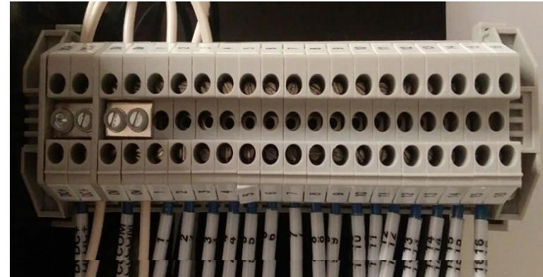
PID Wiring Plate
